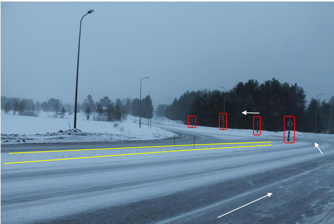
Pos 16/Pic 26. Turning from road 4 toward road 88. Marked signs need to be removed. Marked area need to be filled.
